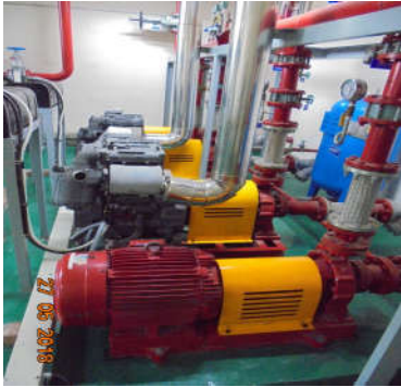
Trạm bơm chữa cháy/ Fire pumping stations
